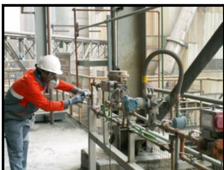
Flow Meter in feeding system
