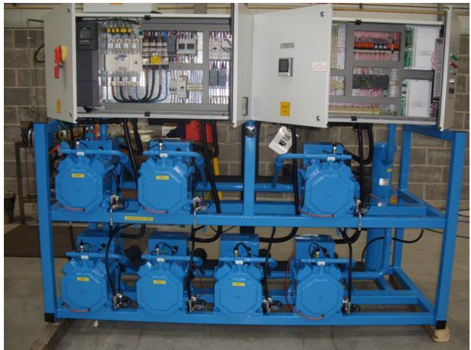
Centralised system: Rack of 7 compressors connected to numerous display cabinets in supermarket and connected to an externally located condenser
