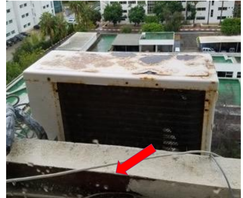
Air Intake Blocked by Roof Beam
