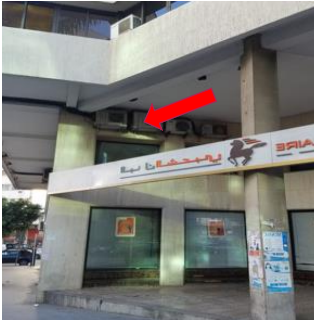
Overhang Obstructs Airflow
