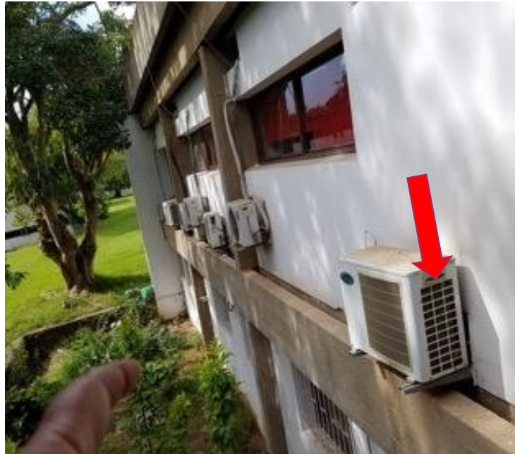
Improper Spacing for Air Intake
