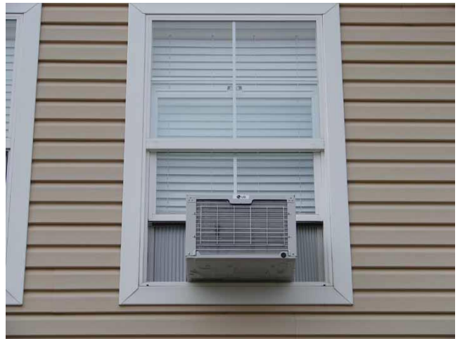
Window mounted air-conditioning unit
