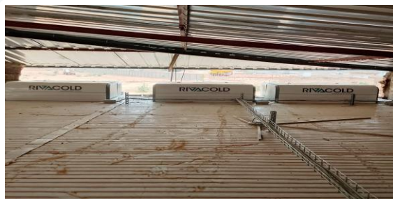
Rivacold R290 monoblocs on roof
