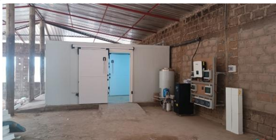
Cold room + pre-room sliding doors
