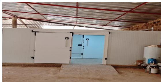
Insulated sandwich-panel cold room
