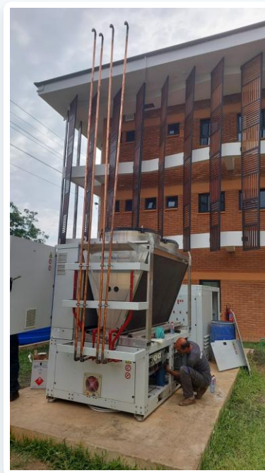
On-site installation — Accra, Ghana
