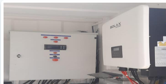
Solax inverter & control panel
