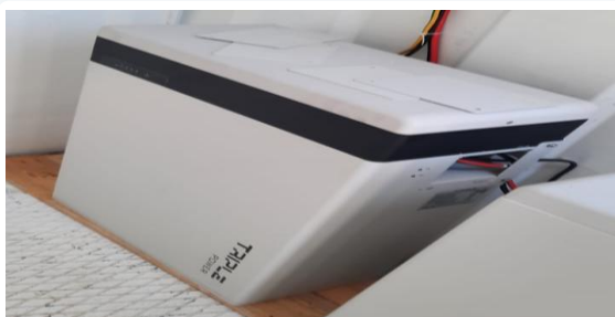
Lithium battery bank
