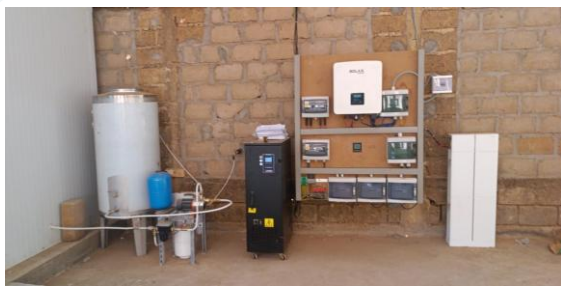
Solax inverter & control cabinet
