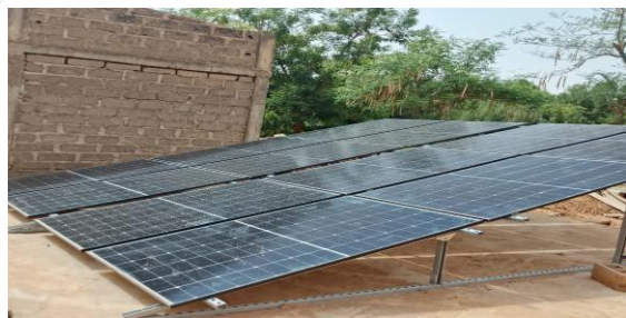
Ground-mounted solar array
