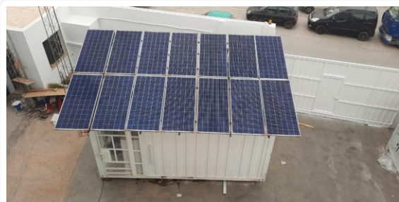
Solar array on container roof
